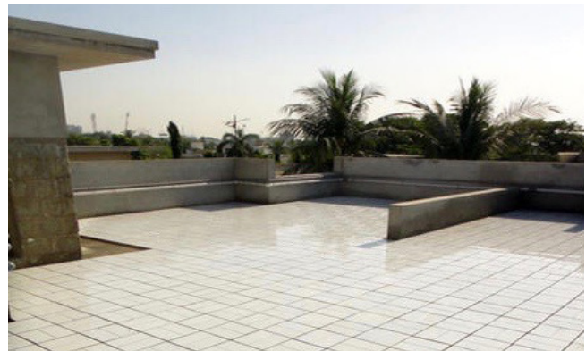
A tiled roof top in the tropics can reflect up to 70% of the sun's heat.
